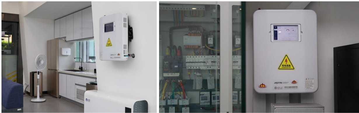
Fig. 10 DC power supply system installed at Tsinghua Sichuan
